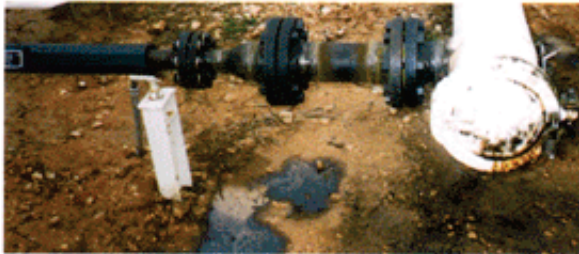
2" Kinetic Cell in 7-mile pipeline, operator eliminated chemicals and reduced pig runs and paraffin to a trace. In service for one year.
