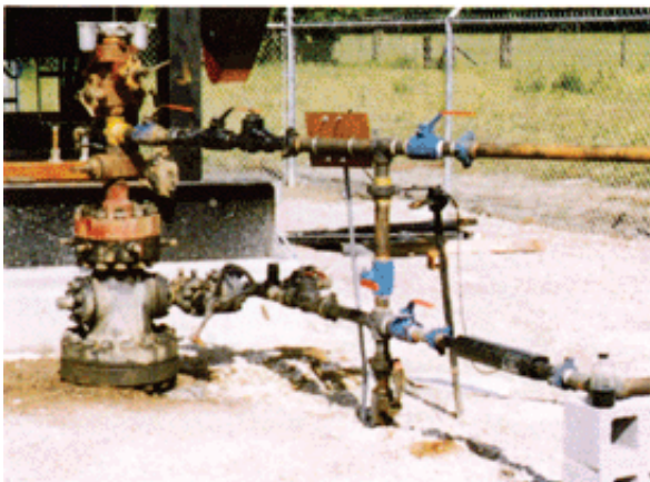
Pumping well in S. Louisiana, 2" tubing, paraffin at 500' daily. Chemical treatment plus hot oil once a month. Installed a Kinetic Cell and eliminated all treatments. In service for nine months.
