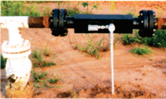
4" Kinetic Cell installed in 4" x 11-mile pipeline, operator eliminated chemicals, disposal of paraffin and reduced paraffin to 1/4 gallon and one pig run per week.
