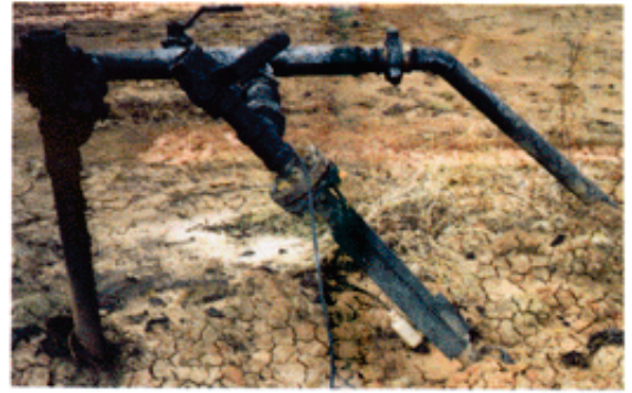
Pumping well in N. Louisiana, 2" tubing, paraffin formed at 500'. Daily chemical treatment, and hot oil once a week. Installed 2" Kinetic Cell at surface, eliminated chemicals, and hot oil once a month. In service for one year.
